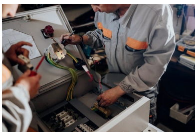
ELECTRICAL TEST PHOTO
